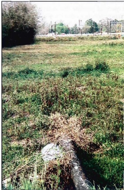
Figure 4: Example of out-of-use pipeline that has migrated to the surface through erosion and other factors.
