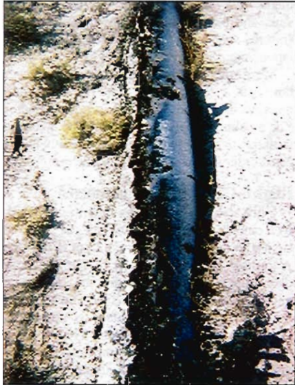
Figure 5: Another example of out-of-use pipeline that has migrated to the surface through erosion and other factors.
