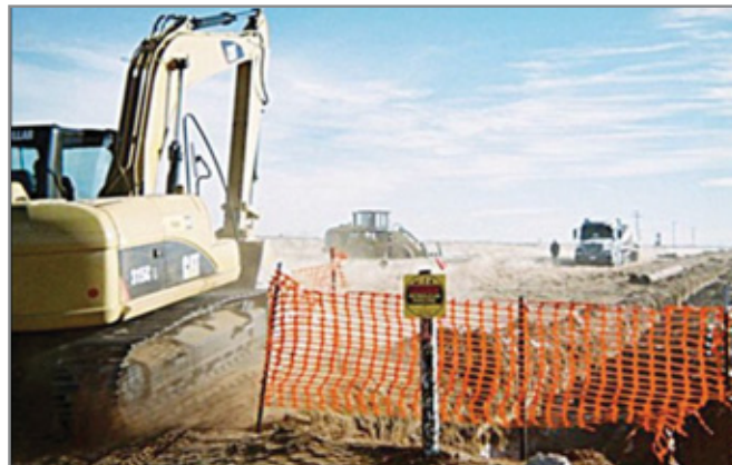
Caution fence at road crossing.
