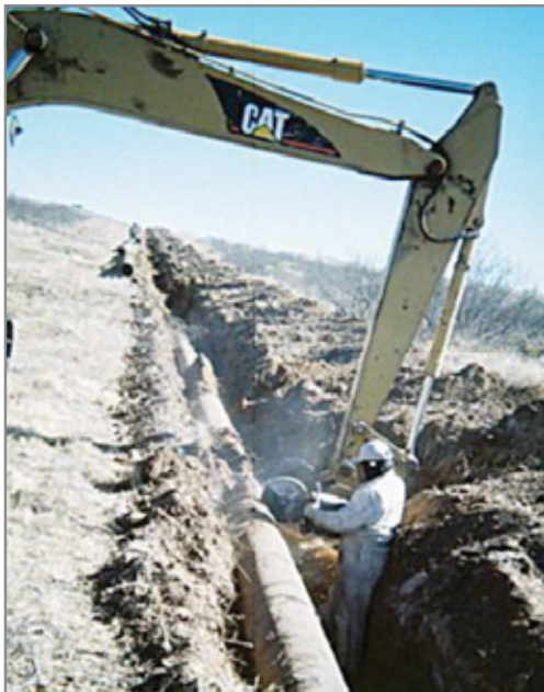
Track hoe lifts pipe to be saw cut. Saws are used instead of torches due to dry grasses in area (fire hazard).
